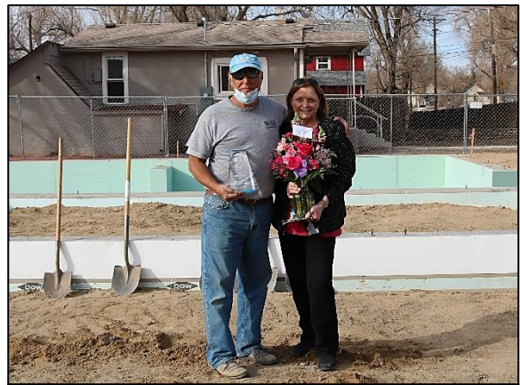
Harry Moore and wife Wanda in front of the foundation of the future “George Hammond Build” house
