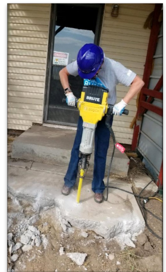
Volunteer Linda Owen uses a jack hammer to make room for a wheelchair ramp
