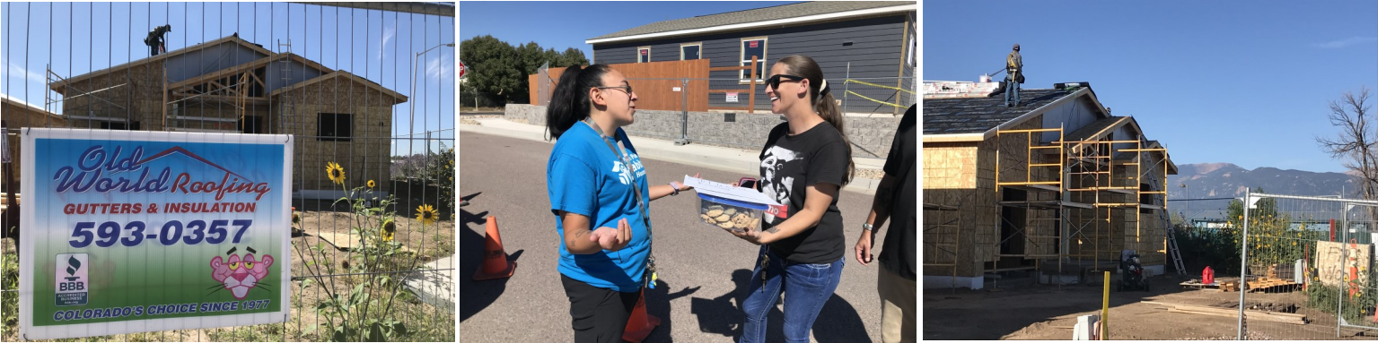
Above left and right, roofing crews work on Bernadette's home on Sept. 23. Above center, future Apostles Build homeowner Bernadette, left, speaks to Tonya Robedeau from Old World Roofing. Bernadette baked cookies and her children wrote thank-you cards for Old World Roofing and GAF.
